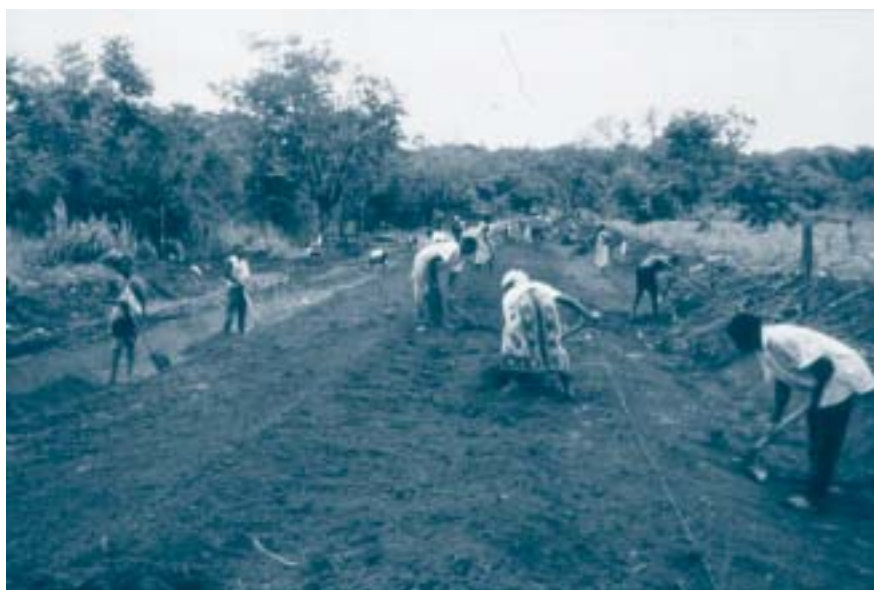
An important objective was to increase local interest within the public and private sectors for sustainably improving physical access for people in rural Zambezia. Measures to achieve this included opting for labour-based methods of road building
